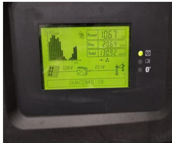
Figure 4: Screen Of Solar Inverter.
